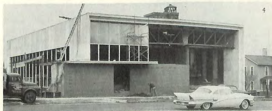
Progress photographs of our new building. #1—excavation, August, 1957; #2—lower level and concrete footing, October, 1957; #3—Steel framing and masonry, February, 1958; #4—Exterior, July, 1958.
